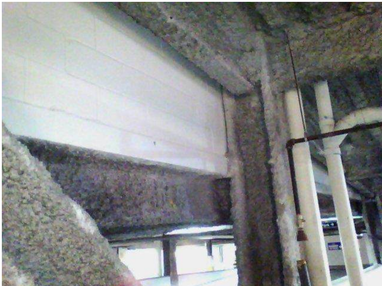
Image FLIR0664. Infrared and visible band images of Location 10 showing evidence of moisture in the insulation.
