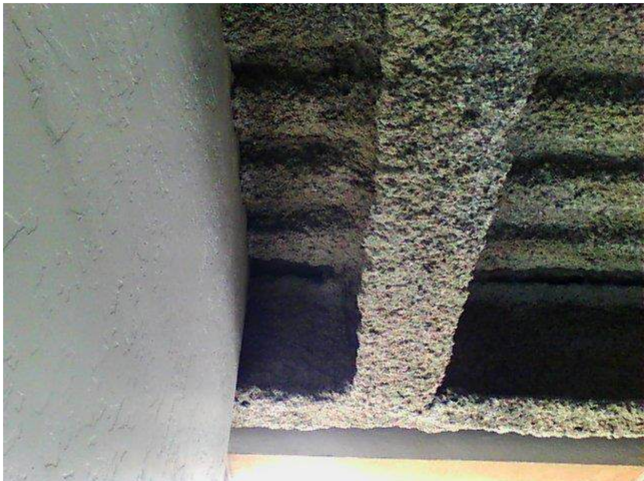
Image FLIR0636. Infrared and visible band images of Location 48 showing evidence of moisture in the insulation.
