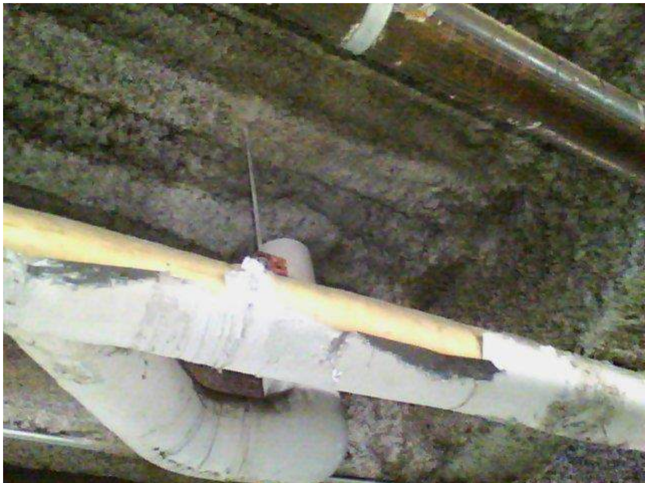
Image FLIR0650. Infrared and visible band images of Location 4 showing evidence of moisture in the insulation.
