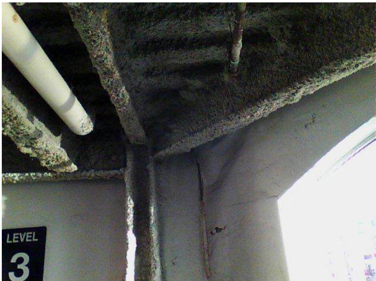
Image FLIR0658. Infrared and visible band images of Location 7 showing evidence of moisture in the insulation.
