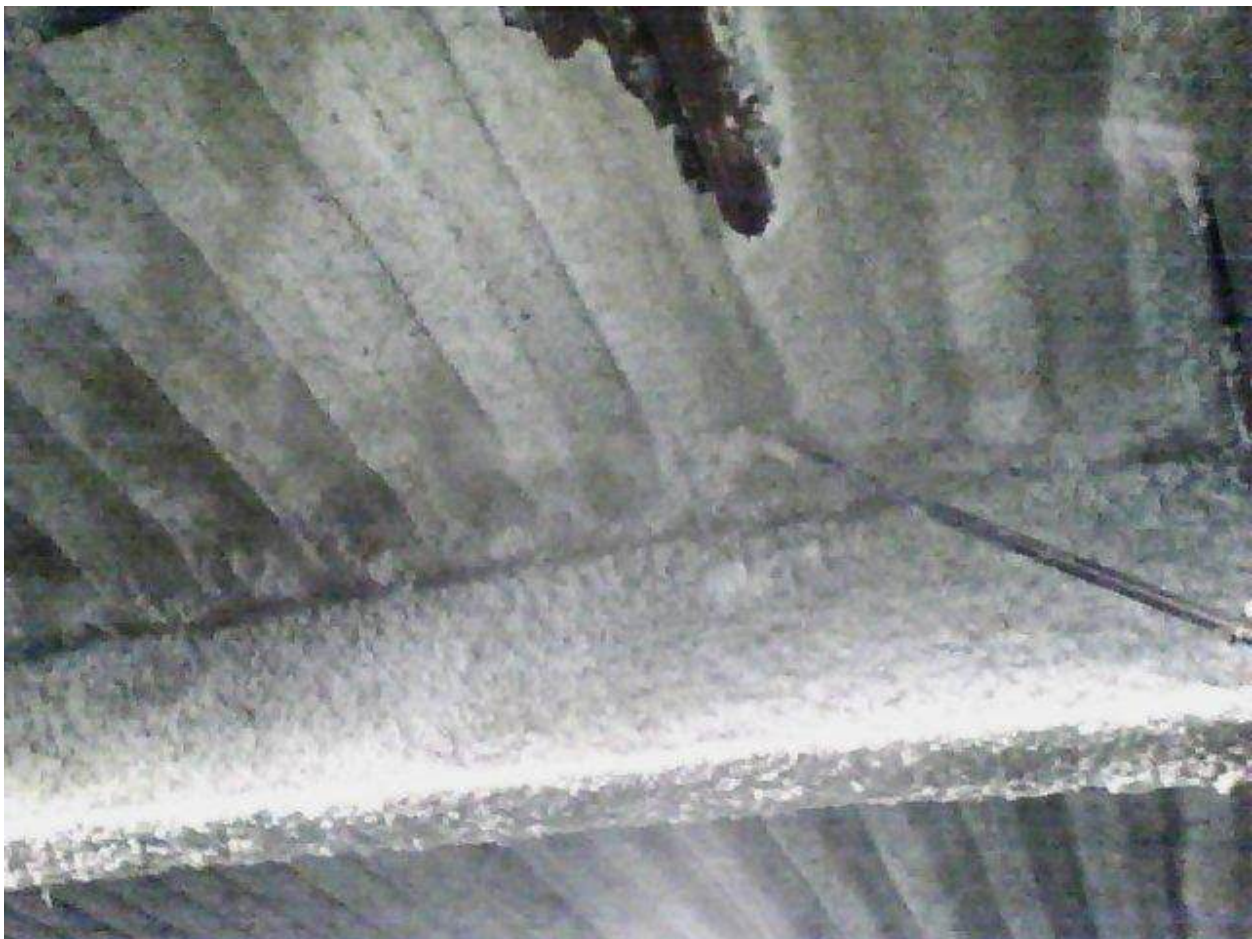
Image FLIR0634. Infrared and visible band images of Location 19 showing evidence of moisture in the insulation.
