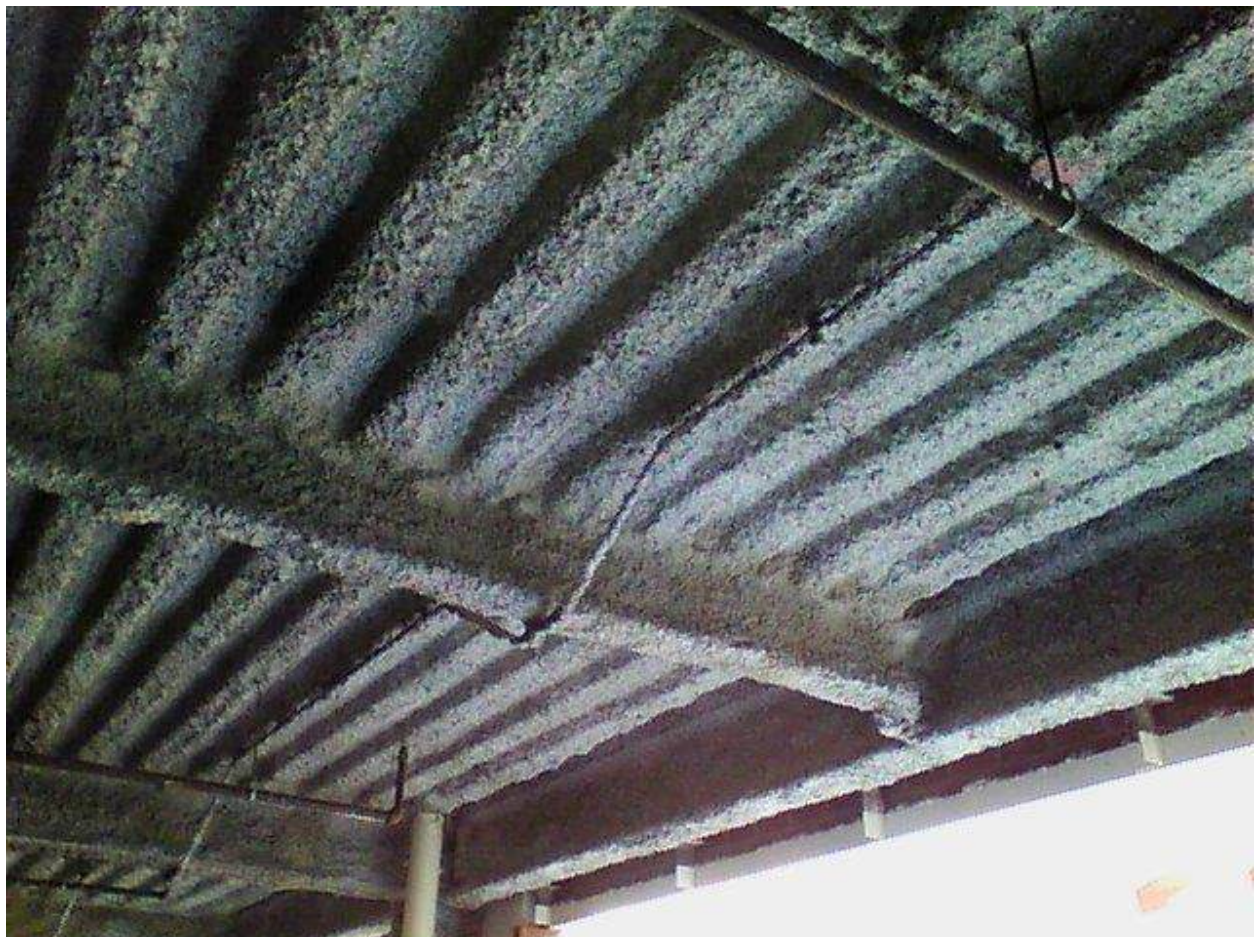
Image FLIR0594. Infrared and visible band images of Location 42 showing evidence of moisture in the insulation.
