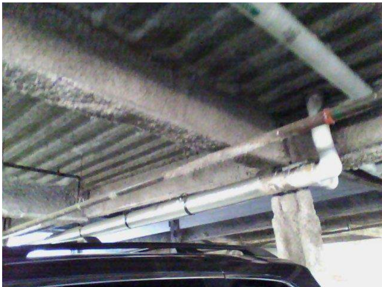
Image FLIR0646. Infrared and visible band images of Location 2 showing evidence of moisture in the insulation.
