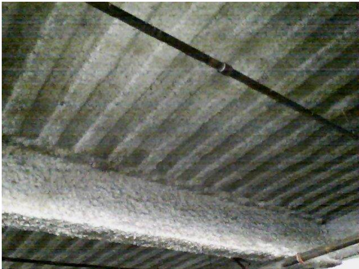
Image FLIR0628. Infrared and visible band images of Location 22 showing evidence of moisture in the insulation.
