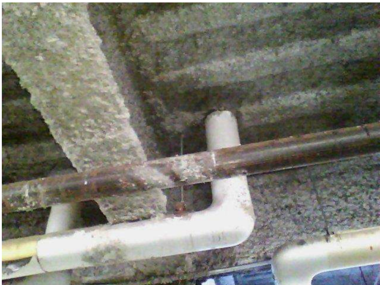
Image FLIR0648. Infrared and visible band images of Location 3 showing evidence of moisture in the insulation.
