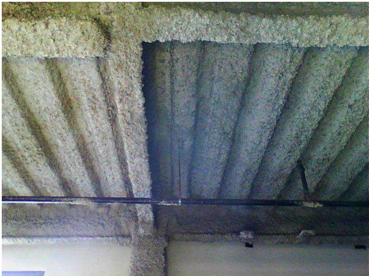
Image FLIR0610. Infrared and visible band images of Location 32 showing evidence of moisture in the insulation.
