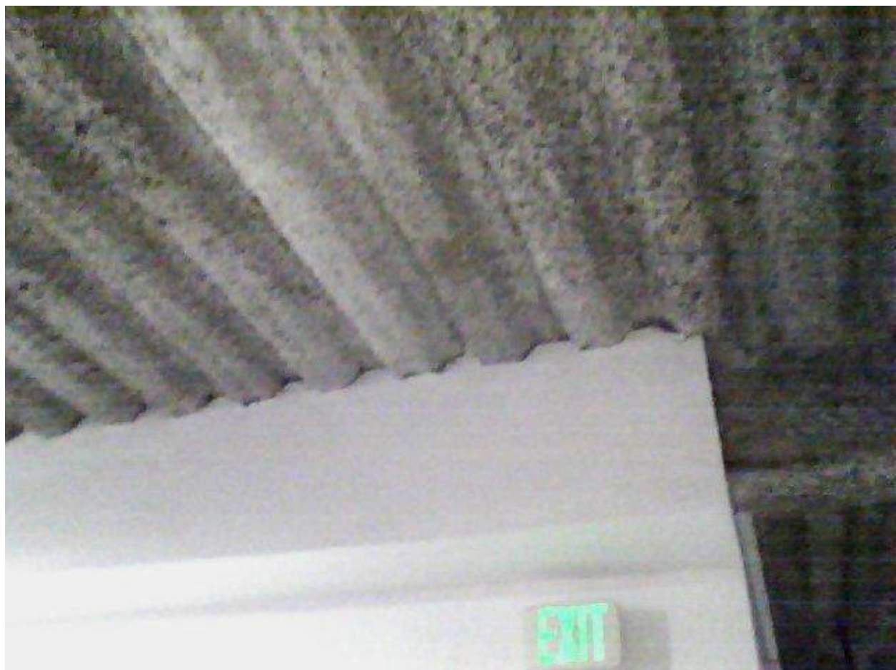
Image FLIR0666. Infrared and visible band images of Location 11 showing evidence of moisture in the insulation.
