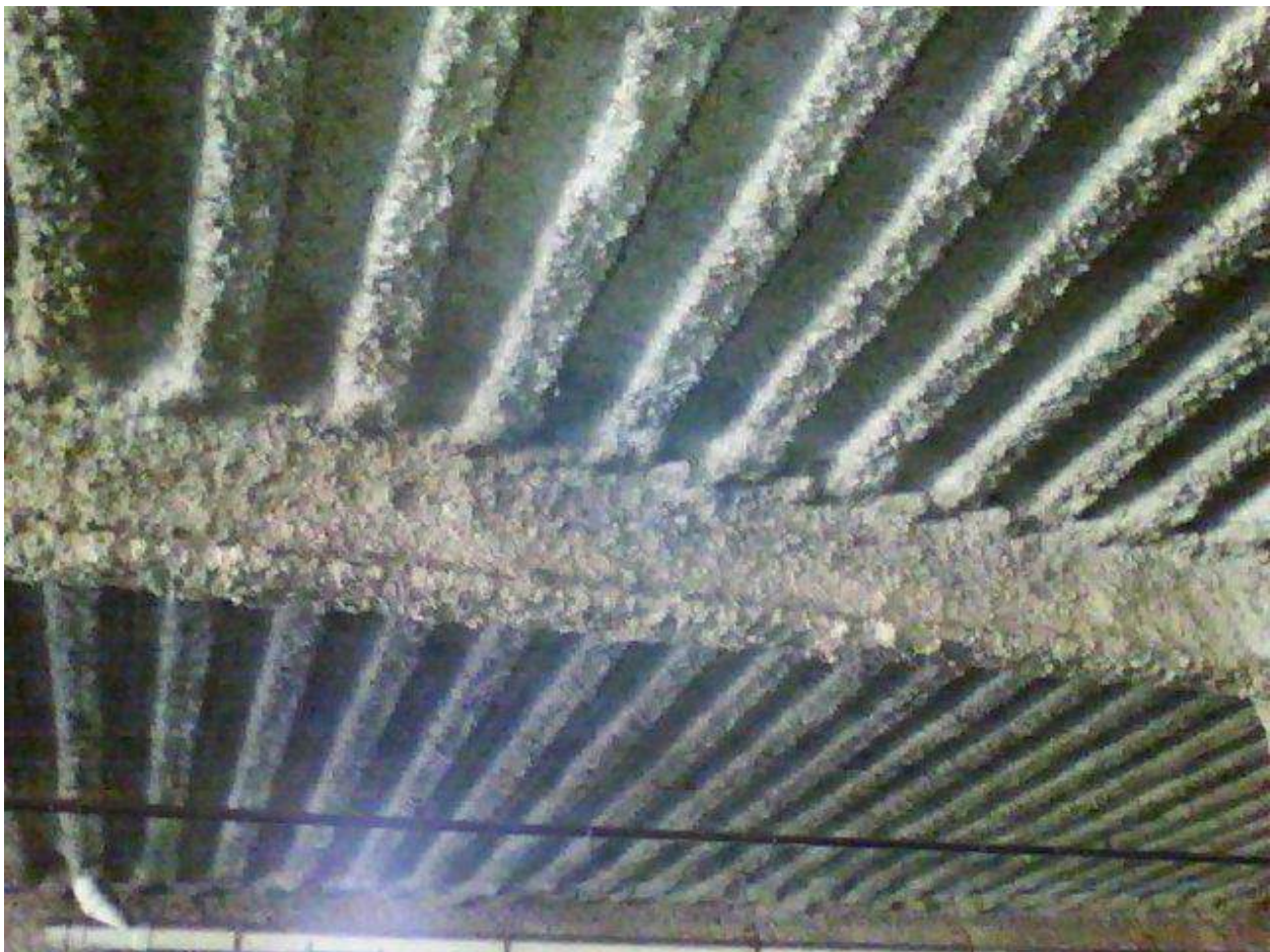
Image FLIR0596. Infrared and visible band images of Location 38 showing evidence of moisture in the insulation.
