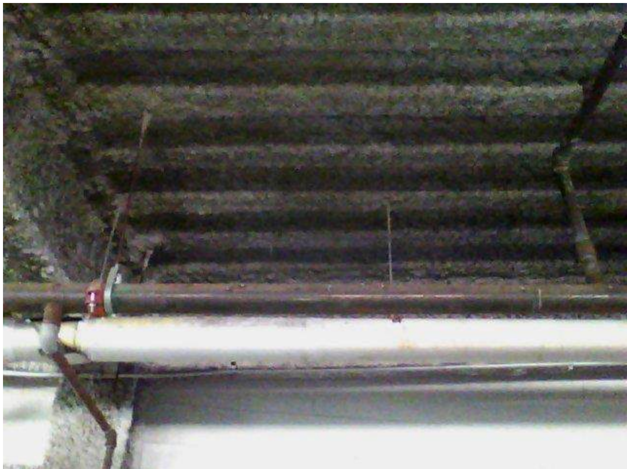
Image FLIR0654. Infrared and visible band images of Location 5 showing evidence of moisture in the insulation.
