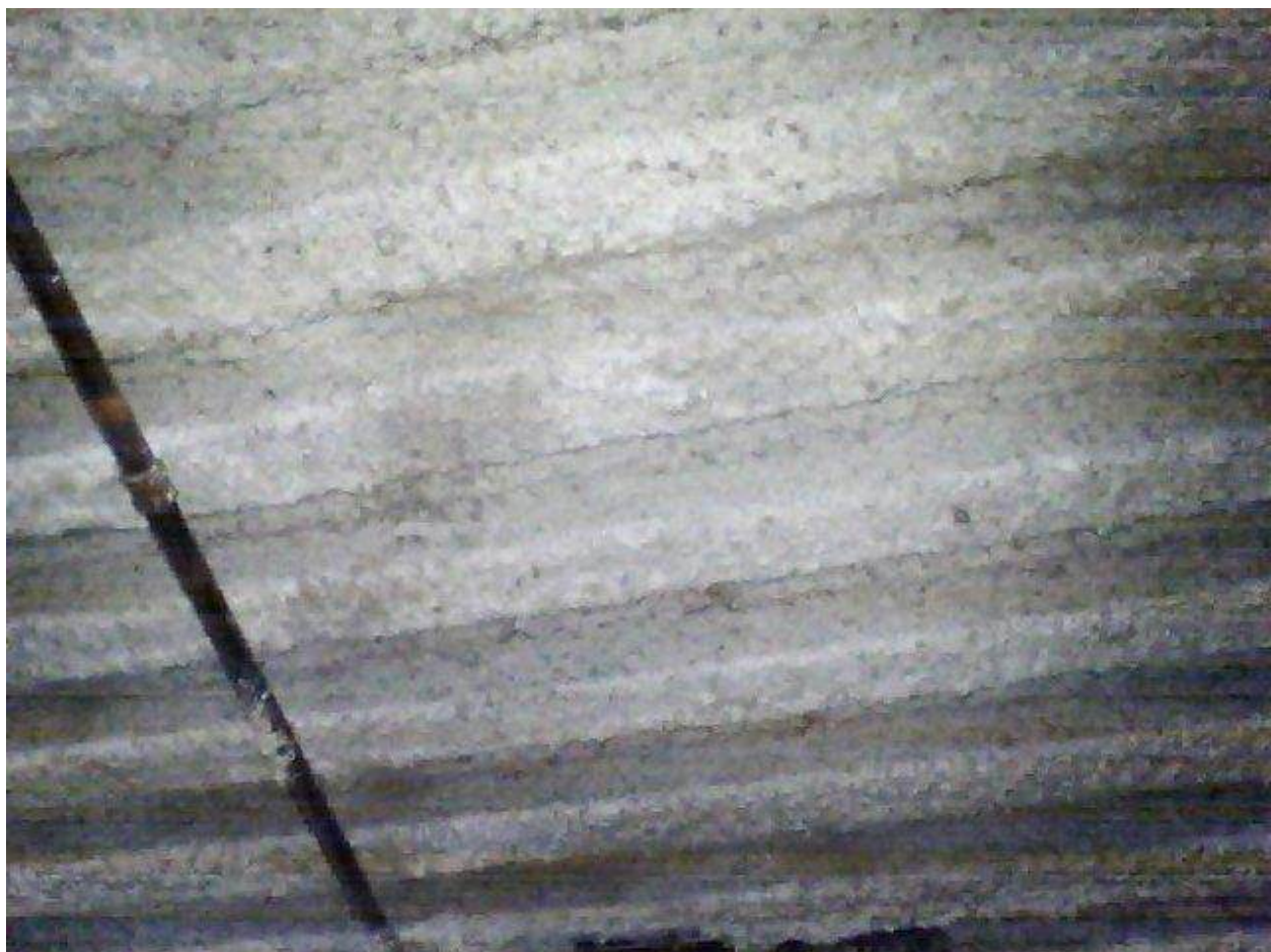
Image FLIR0632. Infrared and visible band images of Location 20 showing evidence of moisture in the insulation.
