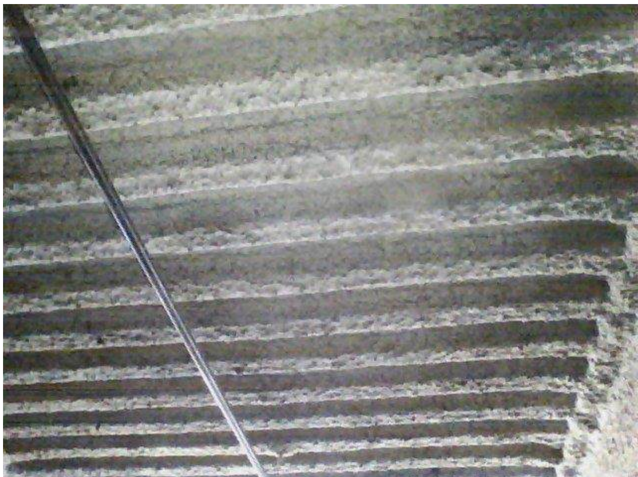
Image FLIR0624. Infrared and visible band images of Location 24 showing evidence of moisture in the insulation.
