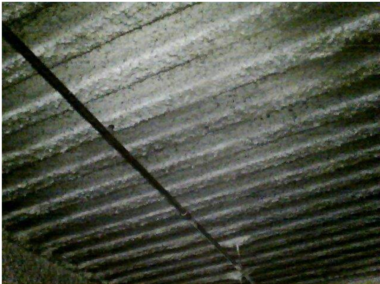
Image FLIR0618. Infrared and visible band images of Location 29 showing evidence of moisture in the insulation.
