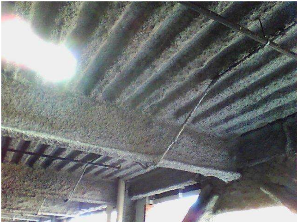
Image FLIR0600. Infrared and visible band images of Location 36 showing evidence of moisture in the insulation.
