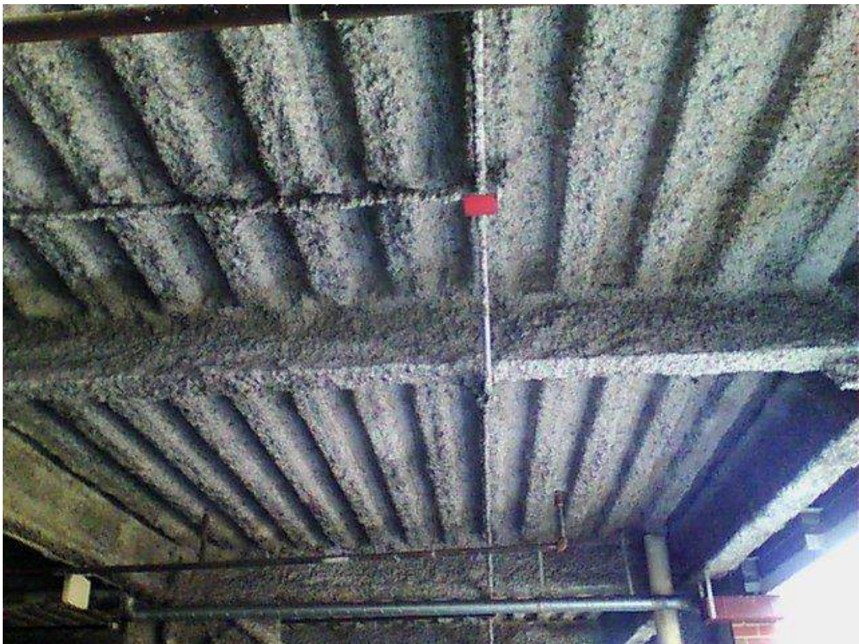
Image FLIR0606. Infrared and visible band images of Location 33 showing evidence of moisture in the insulation.
