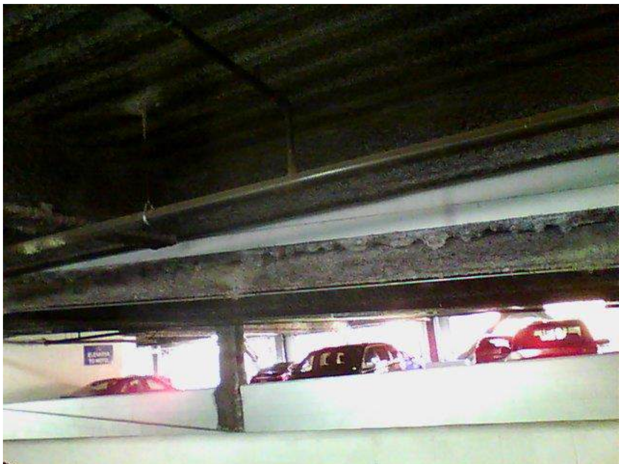
Image FLIR0622. Infrared and visible band images of Location 25 showing evidence of moisture in the insulation.
