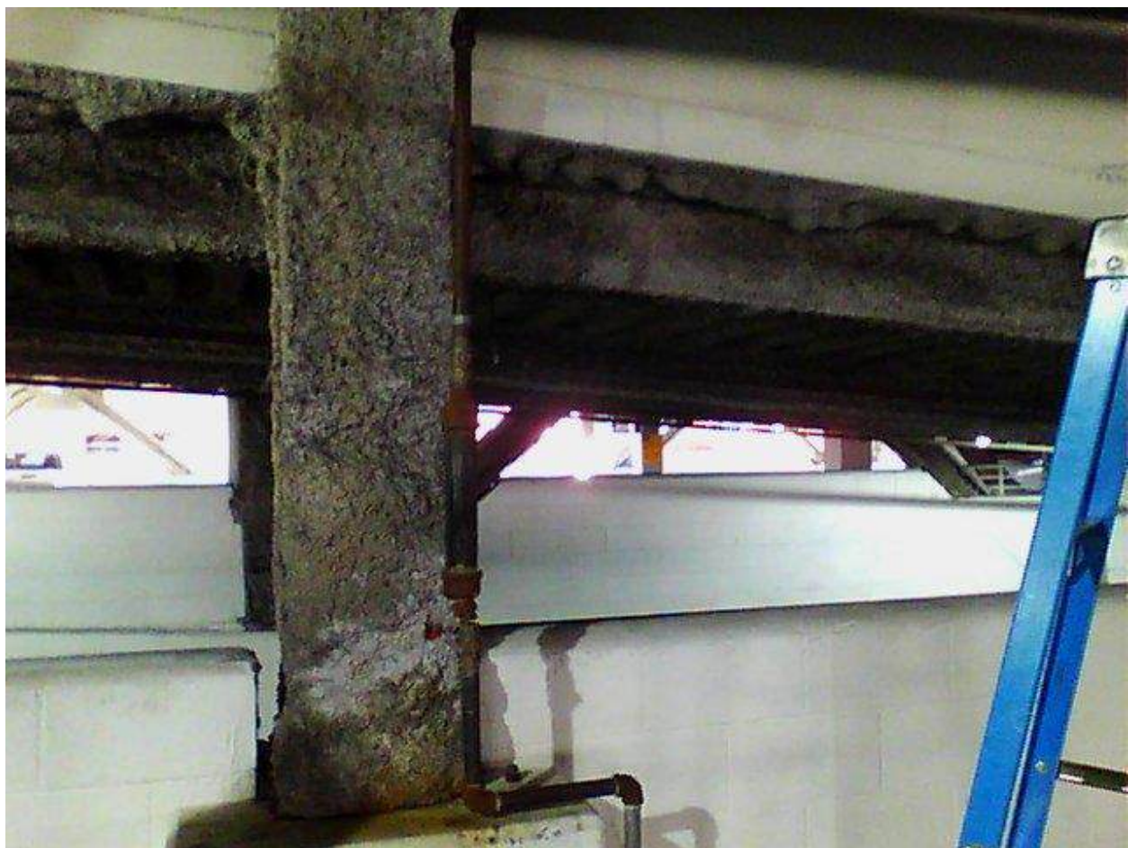
Image FLIR0656. Infrared and visible band images of Location 6 showing evidence of moisture in the insulation.
