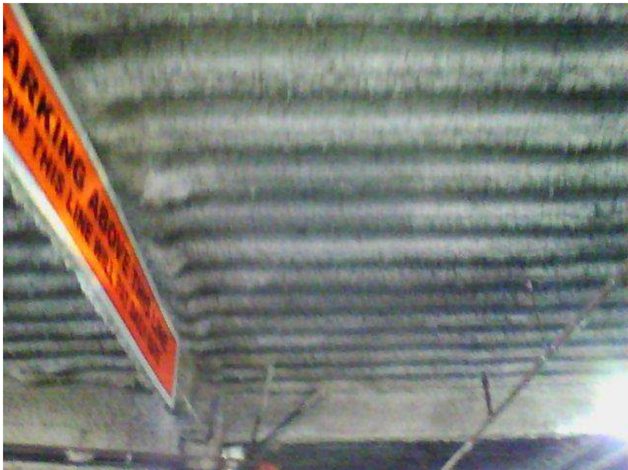
Image FLIR0586. Infrared and visible band images of Location 17 showing evidence of moisture in the insulation.
