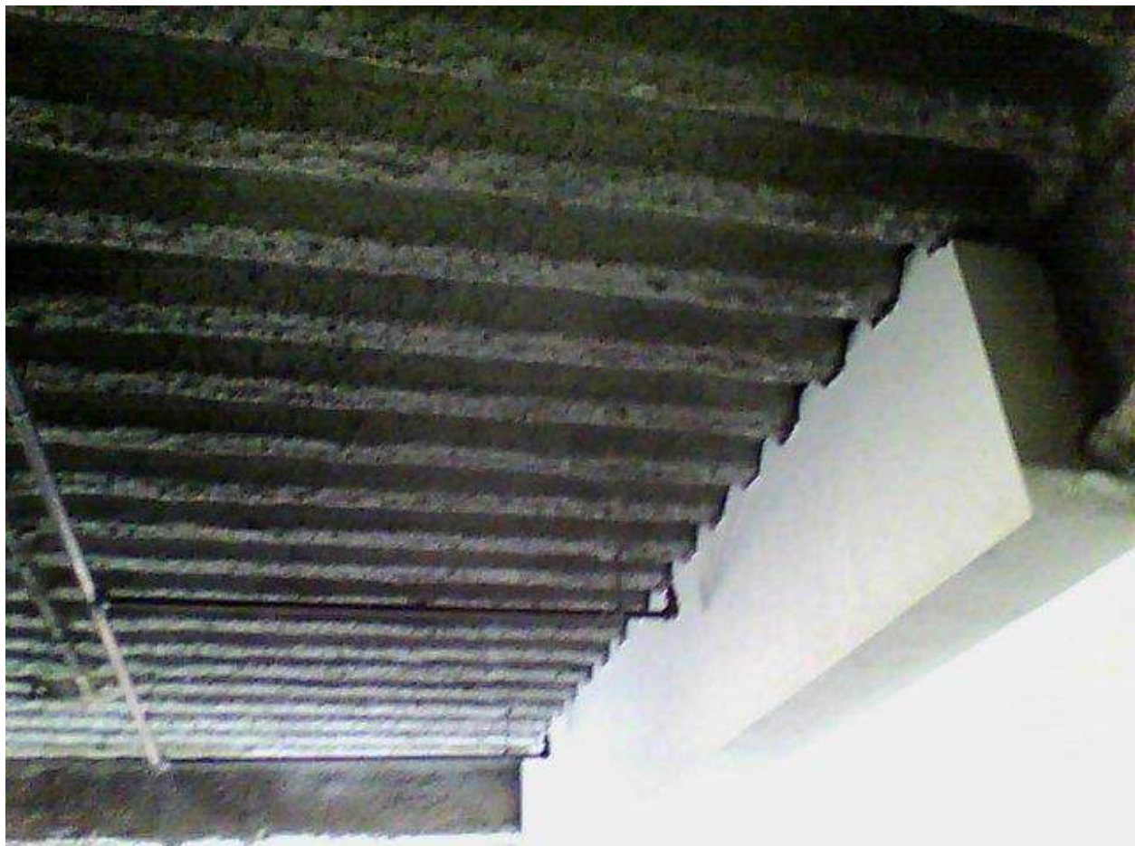
Image FLIR0590. Infrared and visible band images of Location 44 showing evidence of moisture in the insulation.
