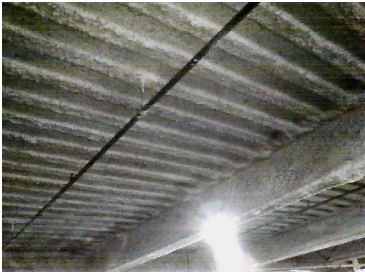
Image FLIR0626. Infrared and visible band images of Location 23 showing evidence of moisture in the insulation.
