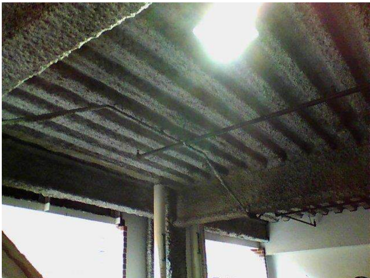
Image FLIR0592. Infrared and visible band images of Location 43 showing evidence of moisture in the insulation.
