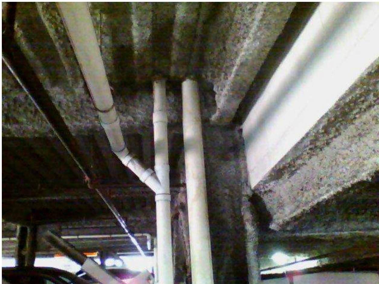
Image FLIR0602. Infrared and visible band images of Location 35 showing evidence of moisture in the insulation.
