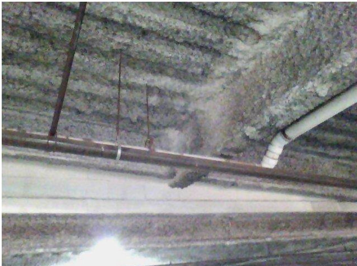
Image FLIR0662. Infrared and visible band images of Location 9 showing evidence of moisture in the insulation.
