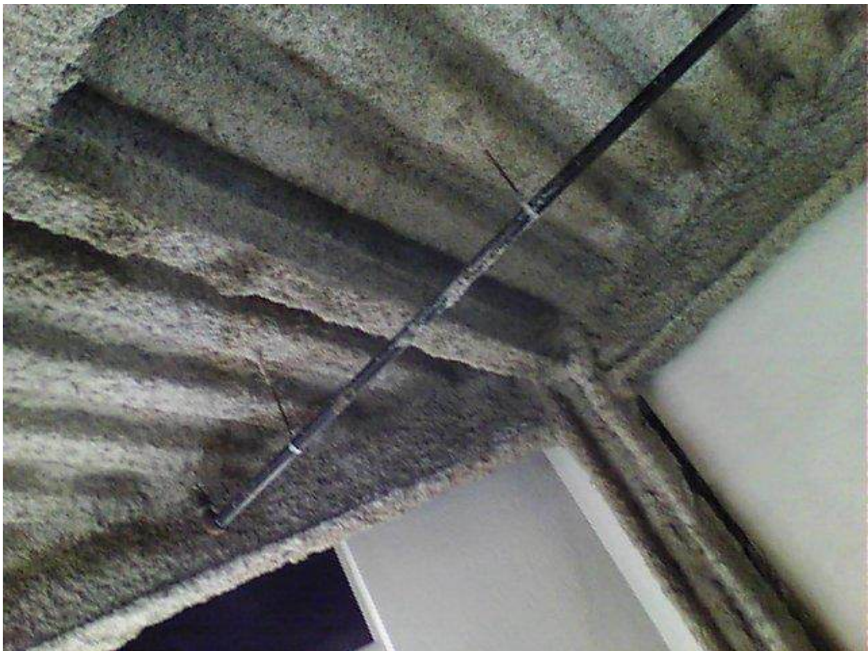
Image FLIR0612. Infrared and visible band images of Location 31 showing evidence of moisture in the insulation.
