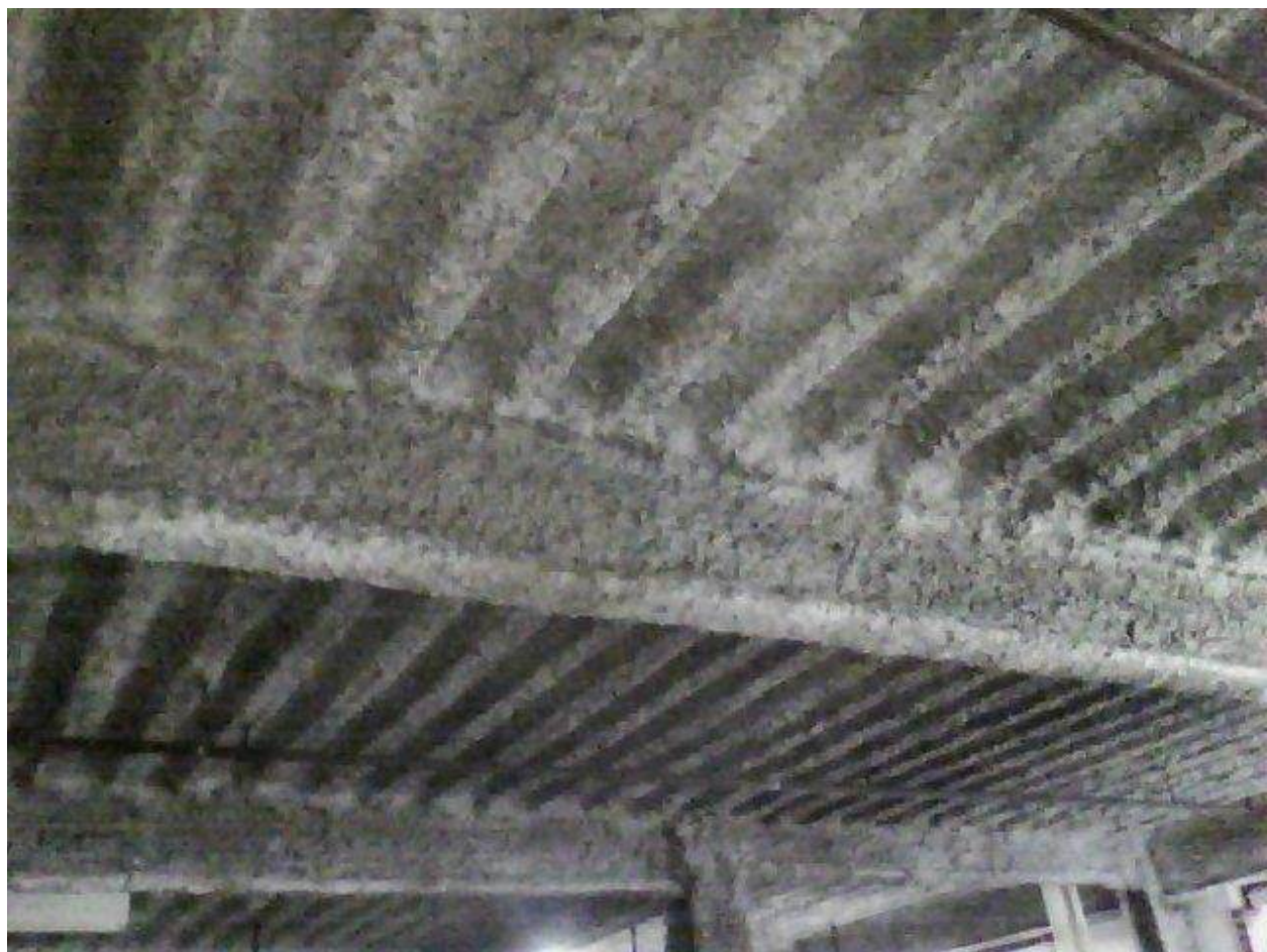
Image FLIR0668. Infrared and visible band images of Location 12 showing evidence of moisture in the insulation.
