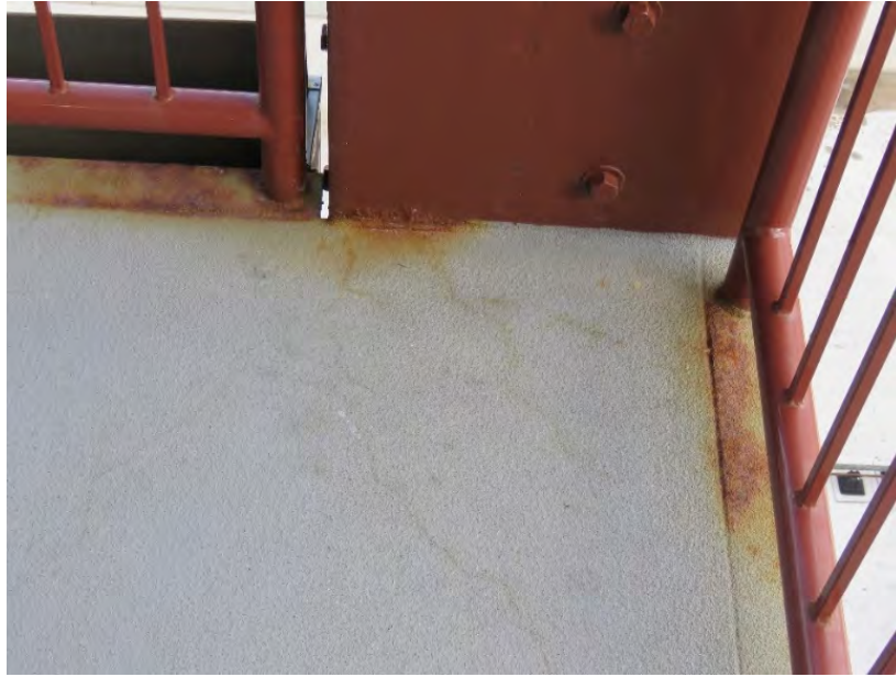
Typical rust and discoloration at handrails throughout facility
