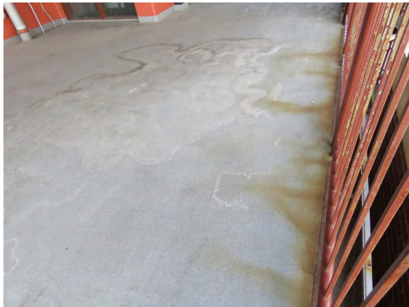
Typical staining at platforms
