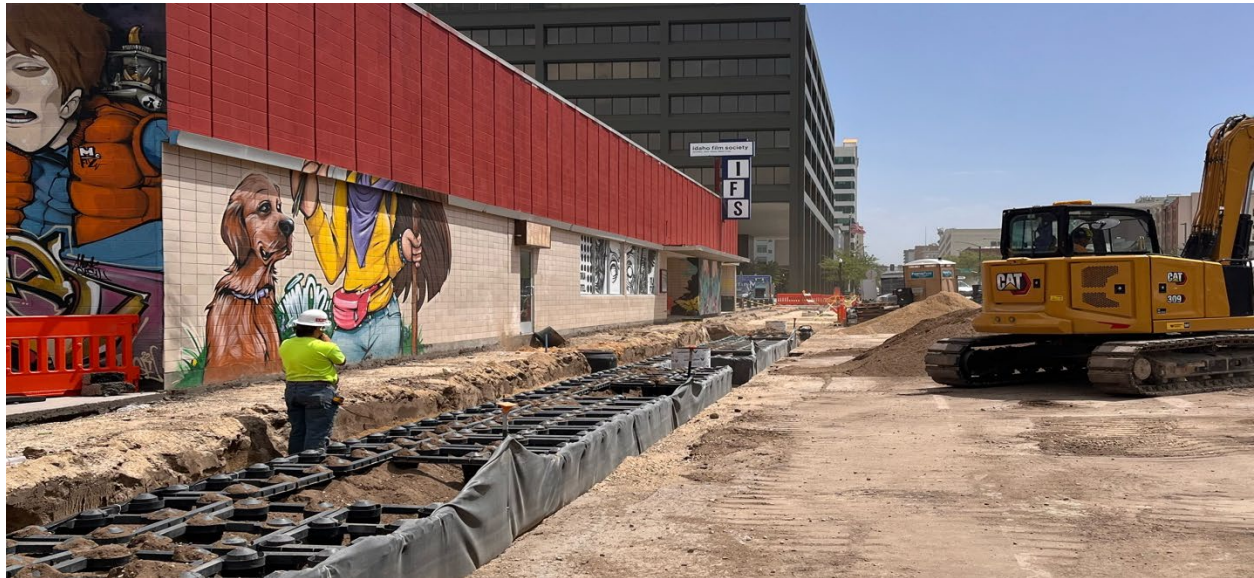
Construction on the Bannock Streetscape Improvements - 12th Street to 16th Street project is underway. Silva cells being installed for the new streetscapes on Bannock Street, in front of the Idaho Film Society building.
