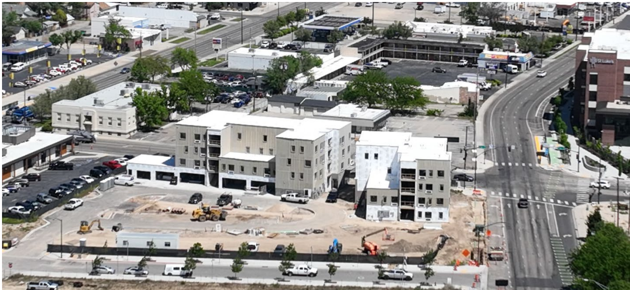
Aerial view of the The Finch, a Type 1 Participation Program partnership with Roundhouse, which is currently under construction
